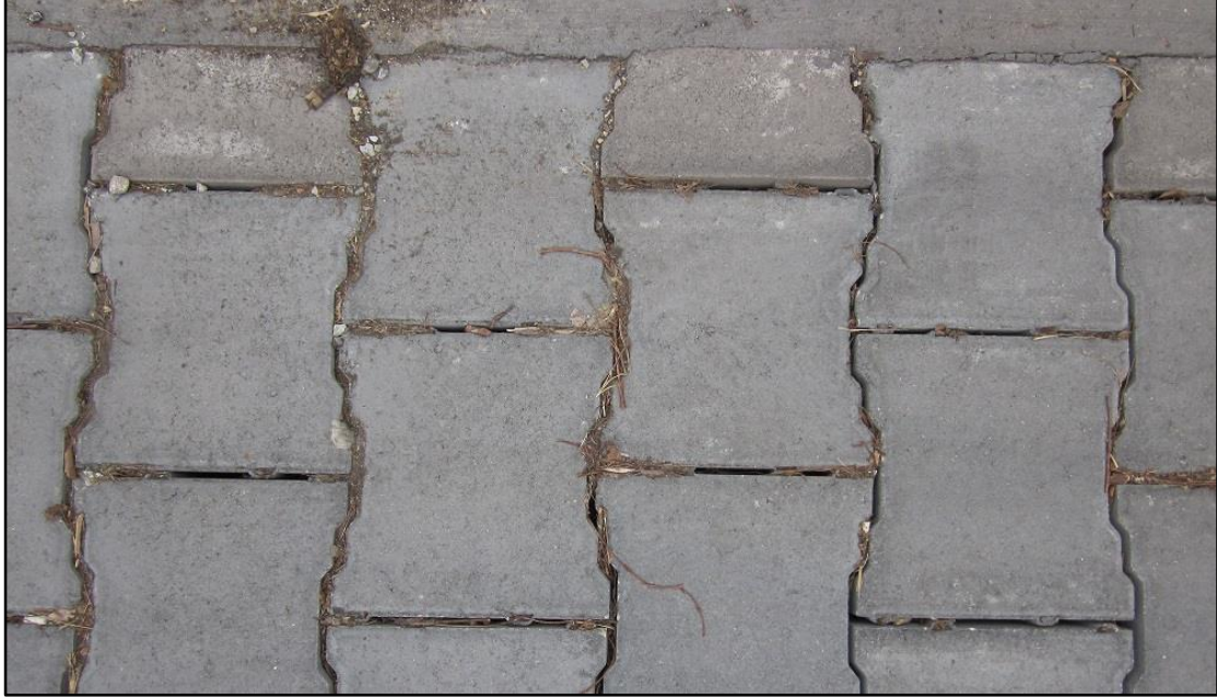
Figure 79 - Observed Surface Clogging on the Surface of Control 19G, February 2012
