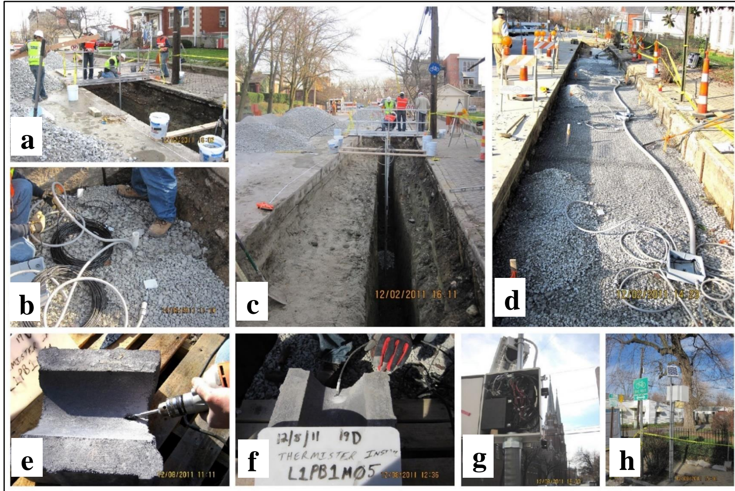
Figure 19 - Installing Sensors in Controls 19G & 19H: a,c) installing piezometer cluster and infiltration tests at the bottom of the trench were conducted from the spanning bridge b) installing surface TDRs d) wires were passed through flexible conduits e,f) thermistor installation g,h) data
